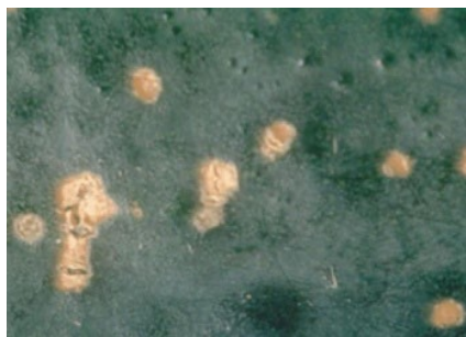
Minor spots on outer surface
